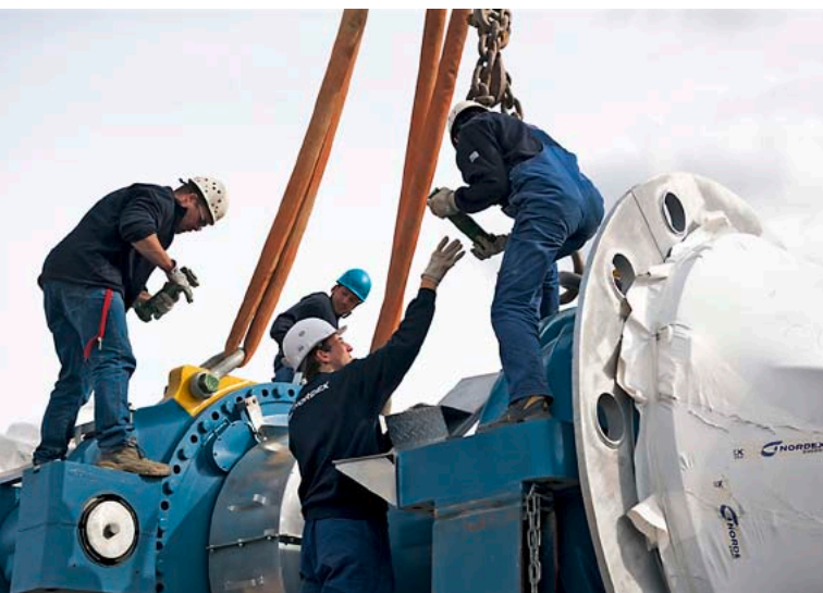
Hétomesnil wind farm, Picardie, France © Wind Power Works
