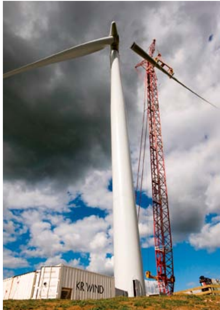
Te Uku wind farm, Waikato © Meridian Energy
