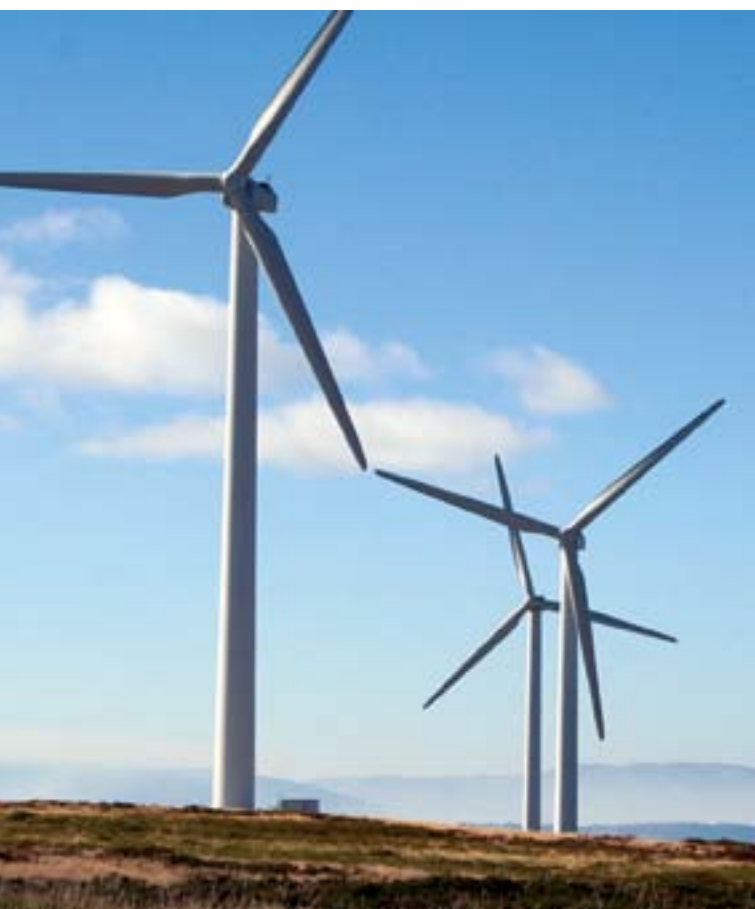
Cabeço Alto wind farm © Nordex Energy
